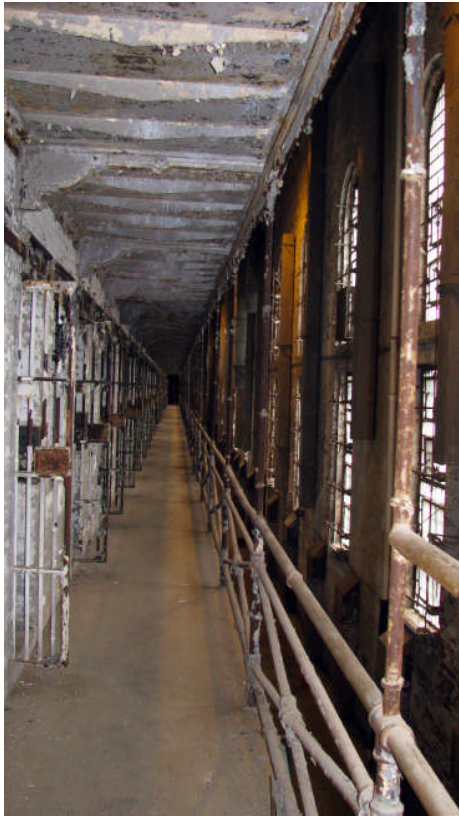
Left: This was taken on the second of six levels on the South side of the West Cell Block. The railings are only thigh high so it was pretty easy for an inmate to either push a guard or another inmate to their death, especially on the sixth level. Christine B. © 2011
